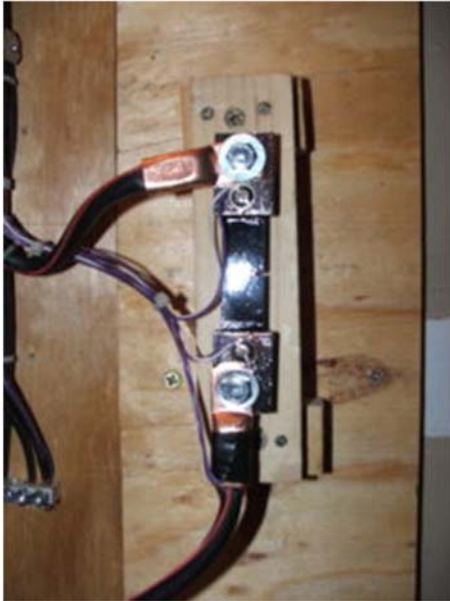
This 100 amp shunt drops only 100 millivolts. The 22 gauge wires connect to the monitor device. ORIGINAL PHOTO ©2022 OFFGRIDHAM.COM
